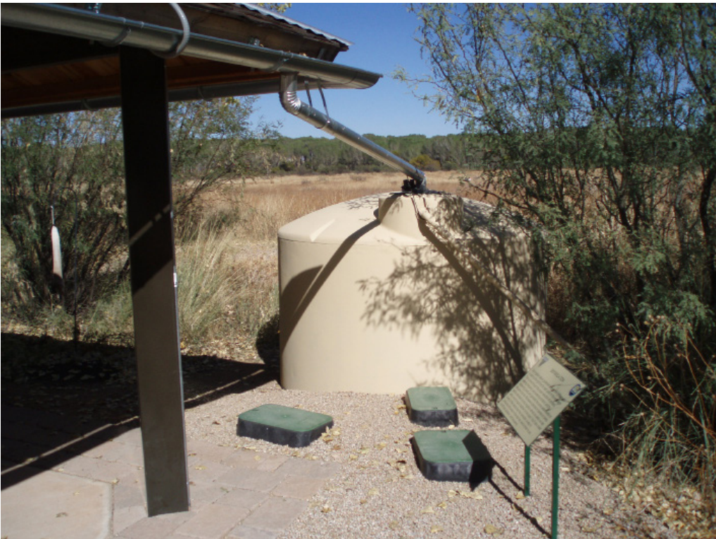
A 1550 gallon rainwater tank supplied with water captured from the roof of the ramada. Note valve boxes protecting the solar-powered pumping system used to water the xeriscape.
